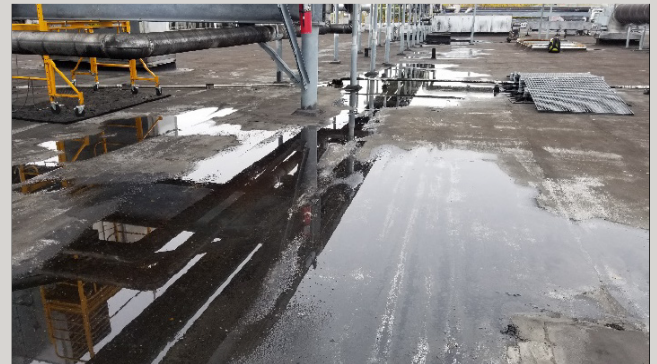
Roof Area B – Partial overview of roof area; ponding water over primary east/west corridor
